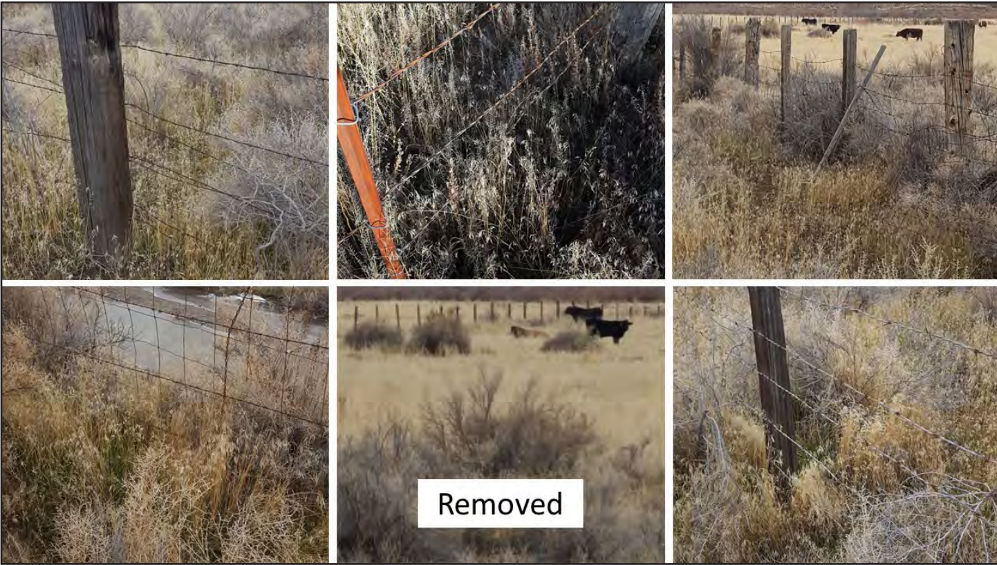
Figure 8. Installation of new fencing using wildlife friendly designs and materials including pipe rail steel fencing which is durable and facilitates ease of movements.
