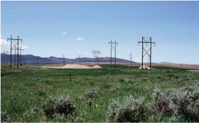
Figure 19. Fences and power lines not only serve as perches for raptors and corvids, but also present a potential collision risk for grouse. (Photos by R. W. Hoffman/retired CPW).
