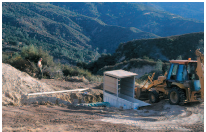
Figure 30. Deer guzzler under construction, San Benito County, California. The collection apron will be installed over the underground storage tanks (left of the access ramp) (Photo by Phil Pridmore/CDFG).
