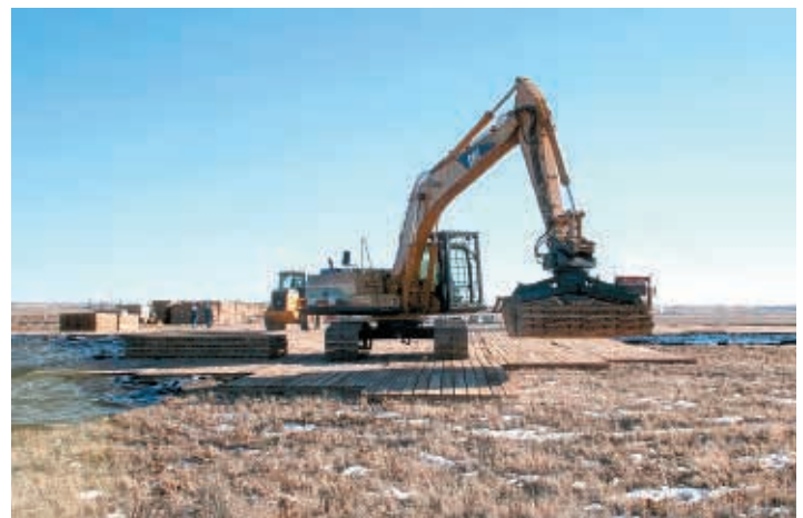
Figure 59. Oak mats being placed directly over drill site to protect top soil. (Photo courtesy of EnCana Oil and Gas).
