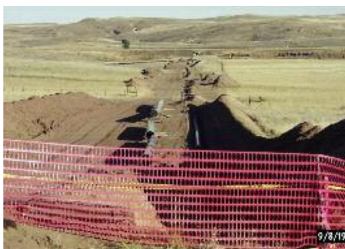
Figure 39. Pipeline construction activities, such as this one in the Powder River Basin, WY, destroy existing habitat, provide sites for invasive species to establish, and temporarily disrupt mule deer movements and use of adjacent areas. (Photo by Bert Jellison/WGFD).
