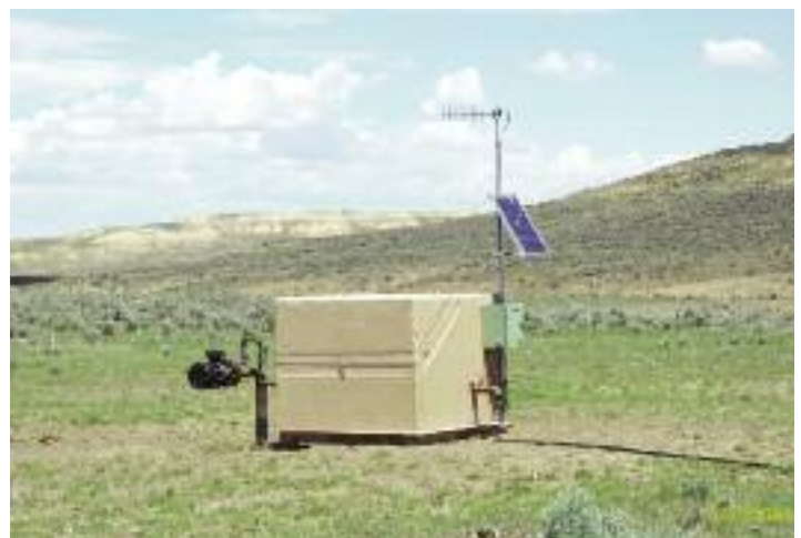
Figure 43. Remotely sensed coal bed natural gas wells in the Powder River Basin, WY have reduced maintenance traffic, which may have beneficial effects for wildlife. (Photo by Olin Oedekoven/WGFD).
