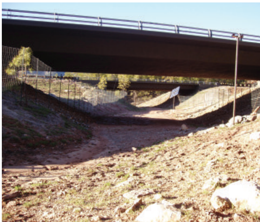
Figure 37. Highway underpass fenced to direct deer safely under the vehicle traffic. (Photo by Norris Dodd/AGFD).
