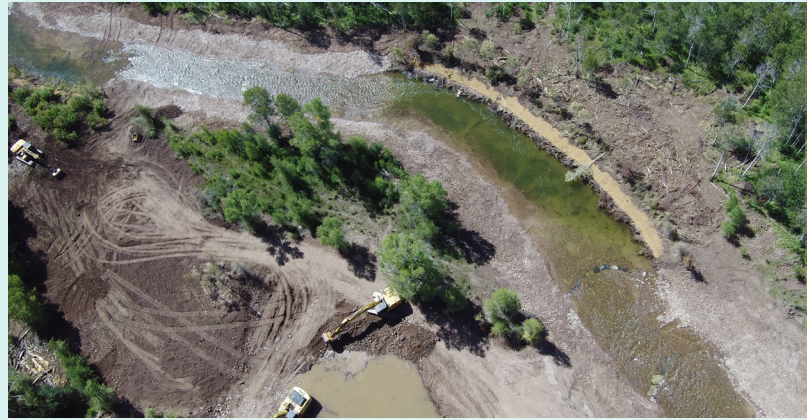
Evanston Town Historic Dam removal during construction. Photo courtesy of Trout Unlimited.
